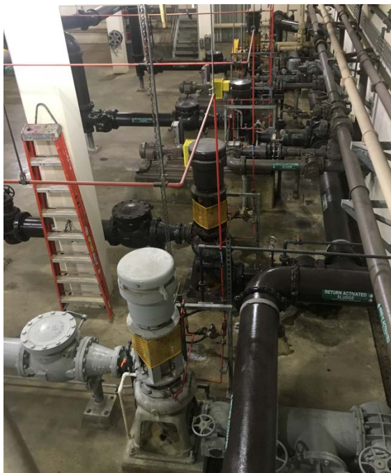
RAS and WAS pumps
