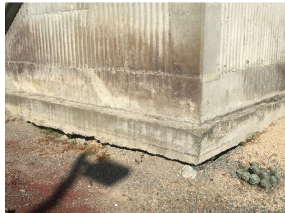
Exposed bottom of process tank
