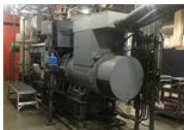
Existing cogeneration system
