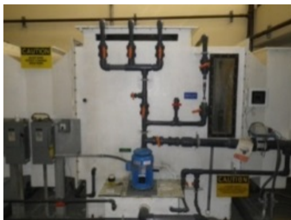
Solids Handling Building odor control scrubber
