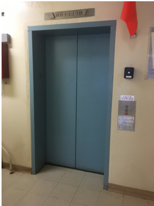
Solids Handling Building Elevator
