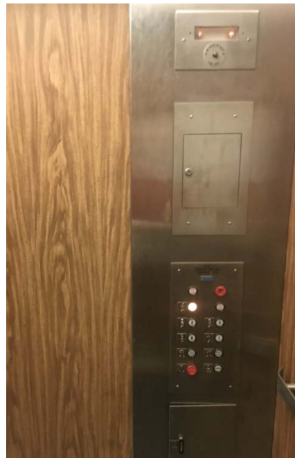
Elevator Control Panel
