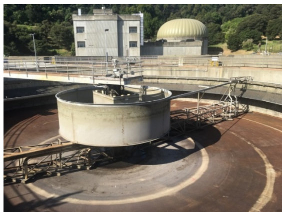
Secondary clarifier internal equipment
