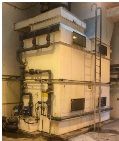
Headworks odor control scrubber
