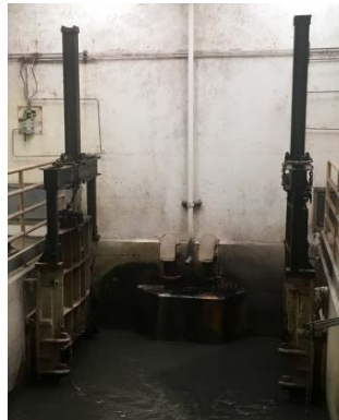
San Rafael and Ross Valley influent gates
