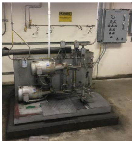
Hydraulic control system
